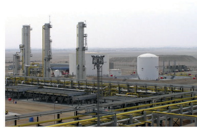
Water purification station
